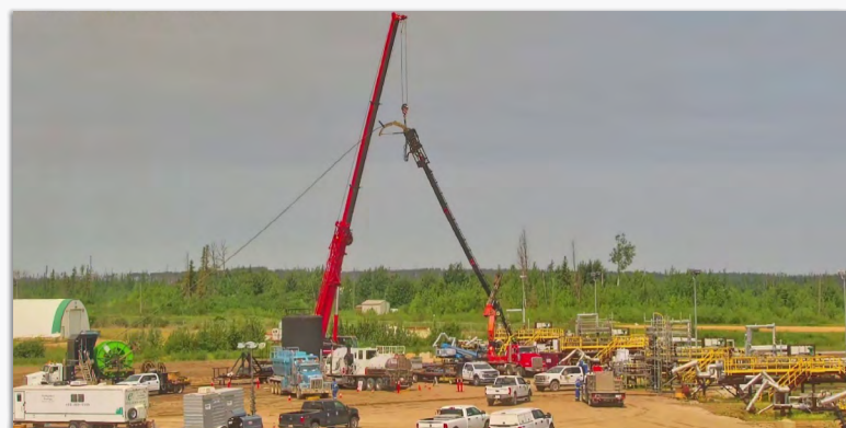
Trial of first coil deployed ESP system in a SAGD well at Long Lake
