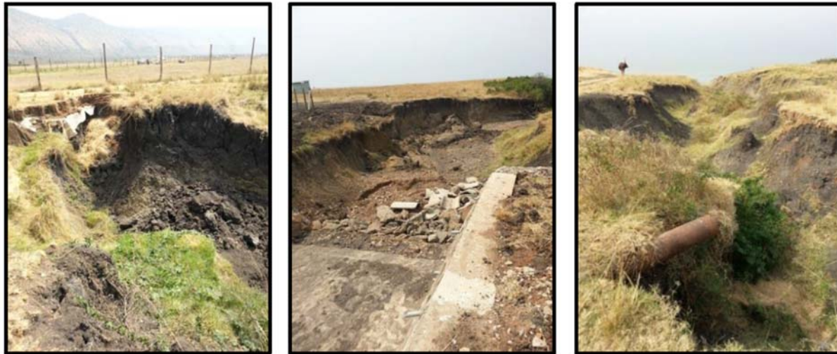
Figure 13: Evidence of soil erosion at the Kingfisher Development Area
