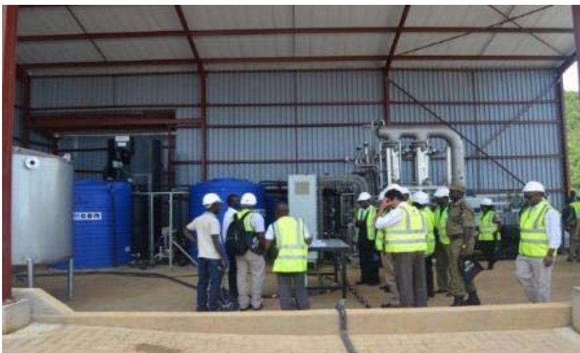
Figure 10: Leachate Treatment Plant at EnviroServ
