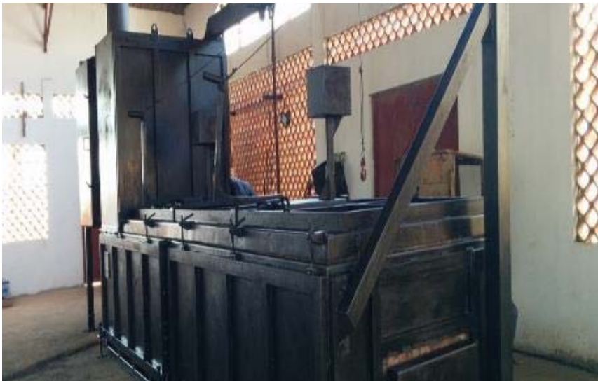
Figure 12: Multiple chamber Incinerator at Green Label's Facility ( www.greenlabelservices.com )
