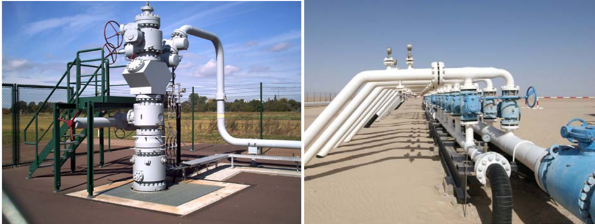
Figure 28: A well head (left) and production manifold (right) (for illustration).
