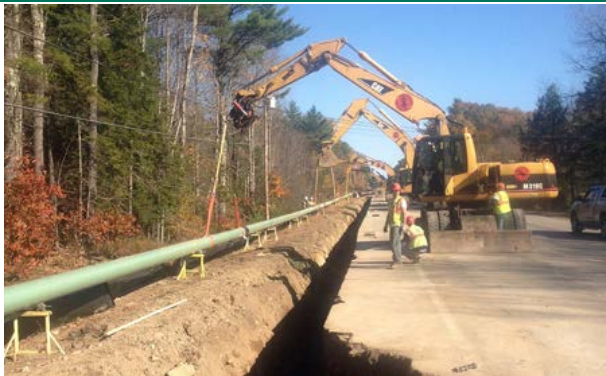
Positioning of a pipeline within a servitude using an existing road as access way
