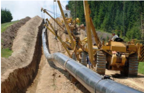
Positioning and lowering of a pipeline along an existing servitude/clearing through a wooded area
