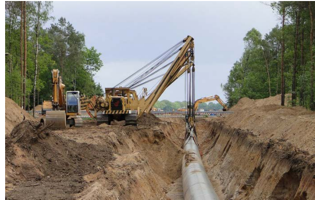
Final placement of a pipeline along a newly created corridor through a wooded area
