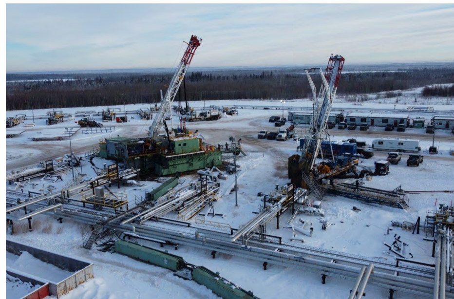
Drilling rig and service rig work in support of our Brownfield program.
